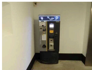
Parking machine in the underground garage
